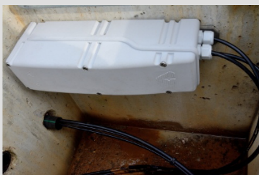
Installation in cable chamber (L1T)
